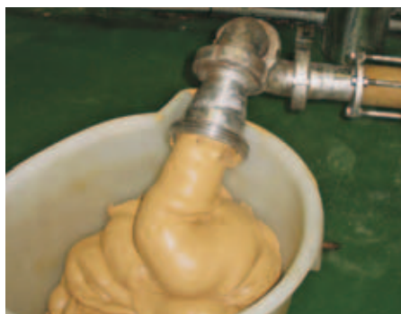
Thick sludge emerges from the STS200 High Performance Solids Management system
